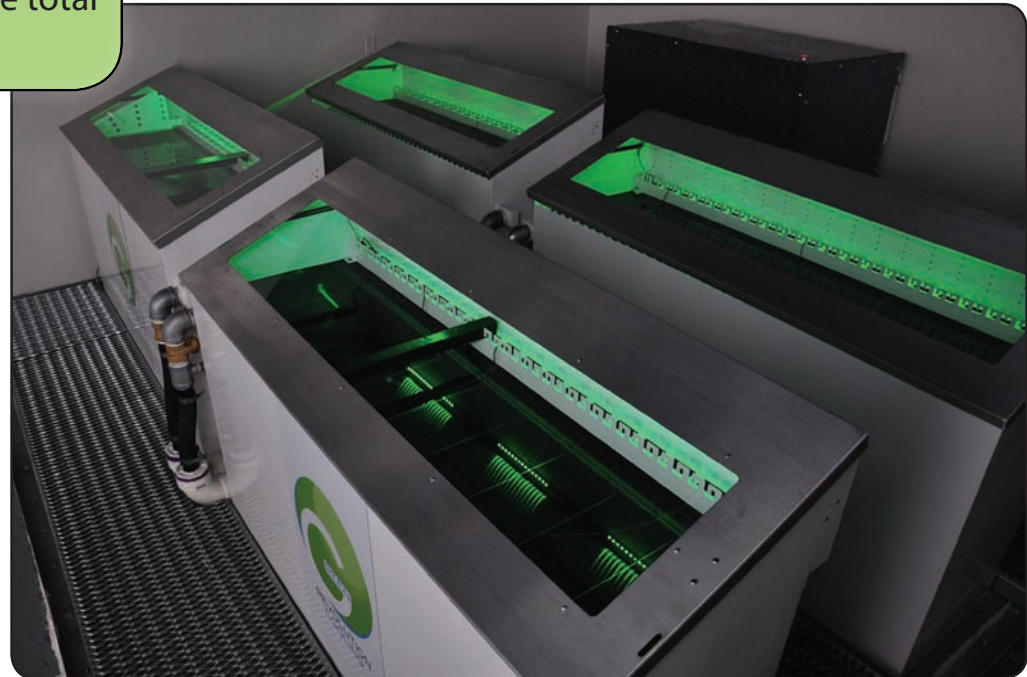
Four-Rack CarnotJet™ System Installation
