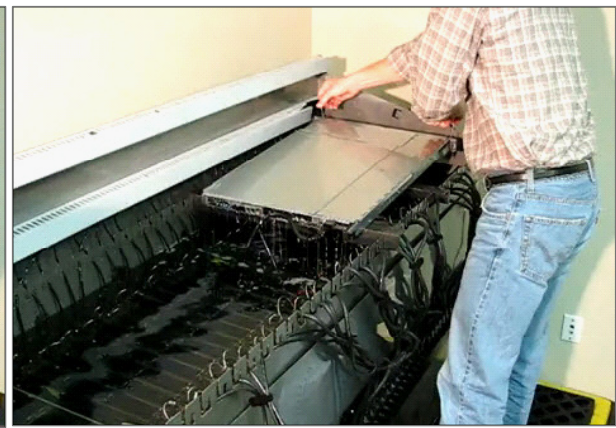
Step 3: Place server on service rails, draining continues
