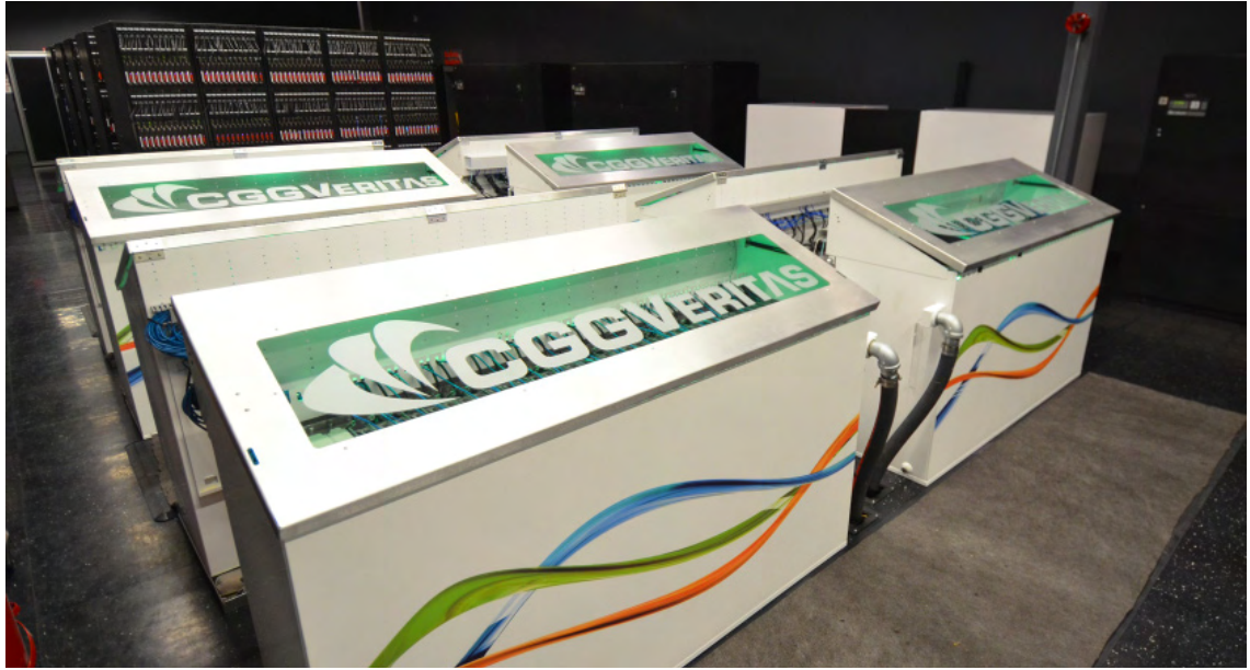
Two CARNOTJET™ system Quads (4 x 42U racks) installed at CGGVeritas in Houston, TX
