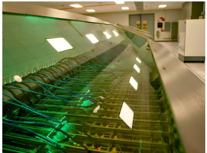
Fig. 4. Network servers are submerged into a tank of mineral oil and hooked up to a pump that circulates the oil. (Photo used with permission from Green Revolution Cooling: grcooling.com.)
