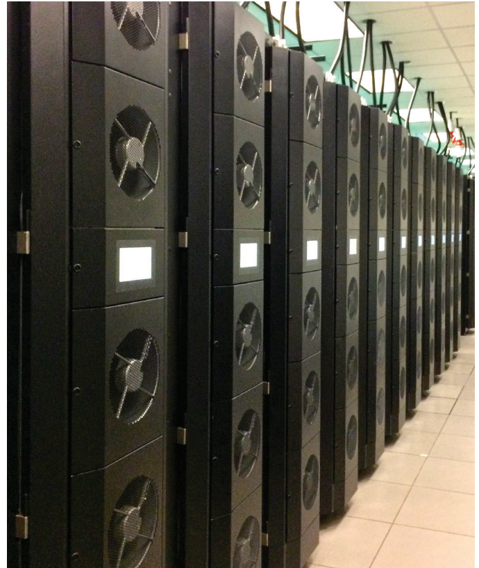
Rear door heat exchangers pull hot air through a radiator, cooling the air in the process, then expell the cooled air back into the data center.
