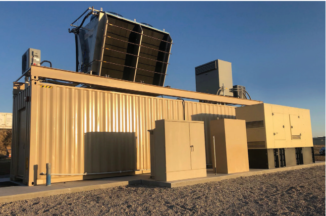
Close to, or far away from civilization, GRC's ICEtank provides a powerful standalone data center that can be placed virtually anywhere power, water and internet is accessible.
