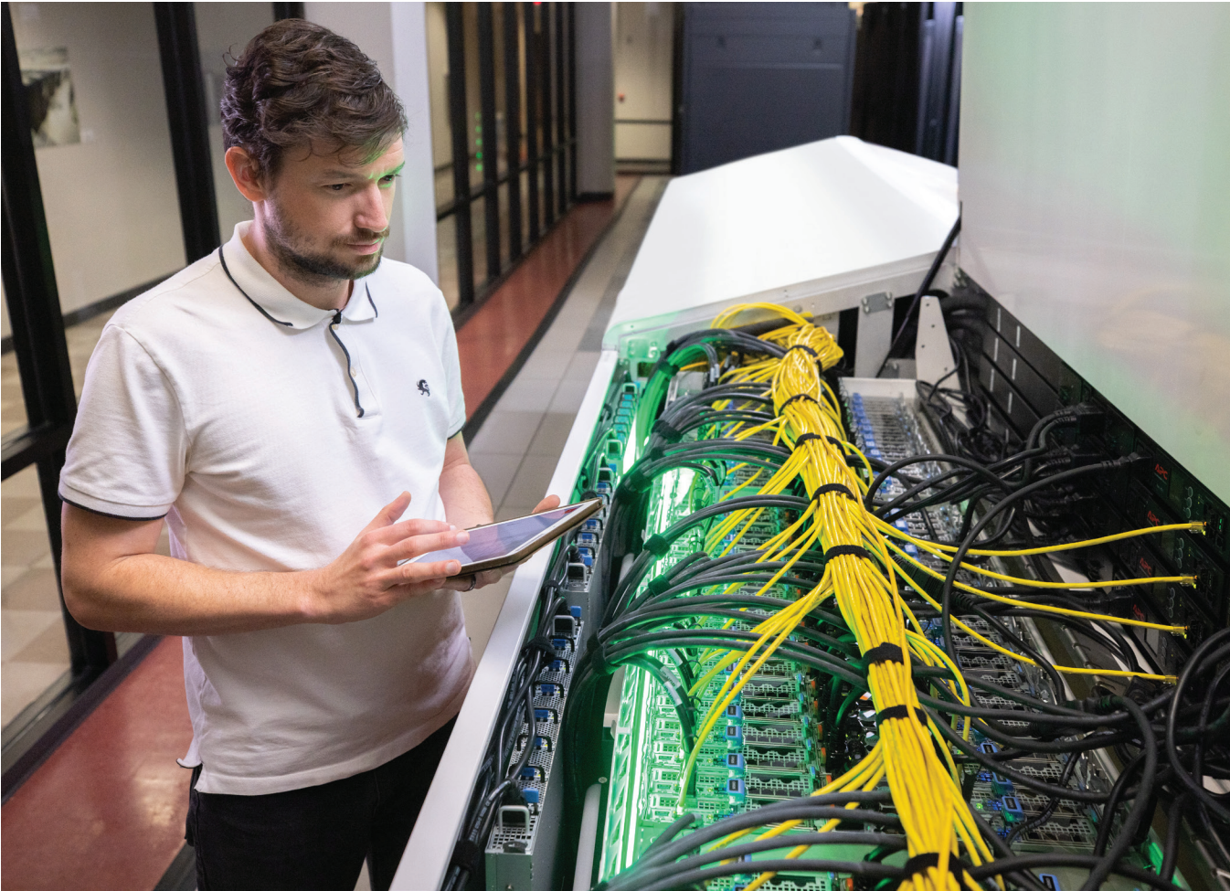
Maintenance on our cooling systems is simple. Servers are easily accessible, and ElectroSafe single-phase immersion coolants do not evaporate like two-phase coolants.
