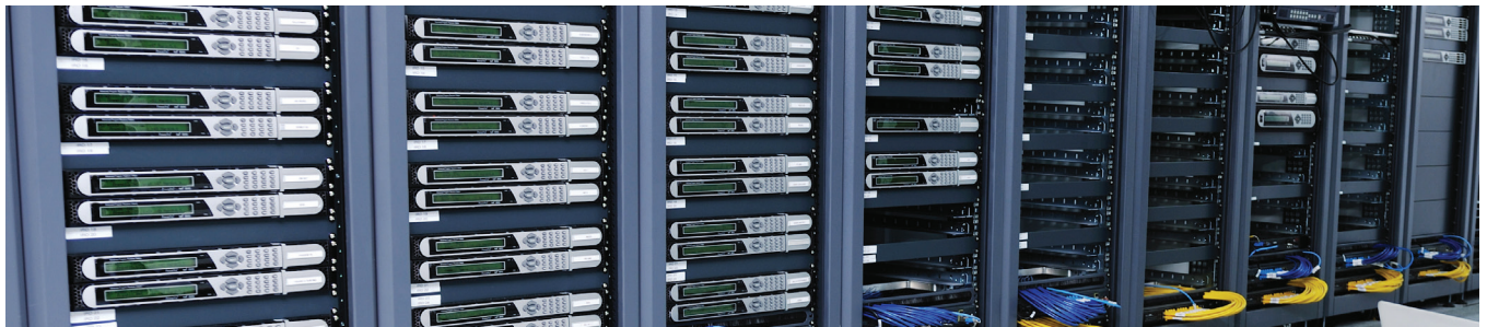
Most air-cooled racks require blanking plates for extra air space between servers
