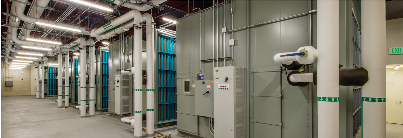
Air handlers and electrical systems for the HVAC in a data center.
